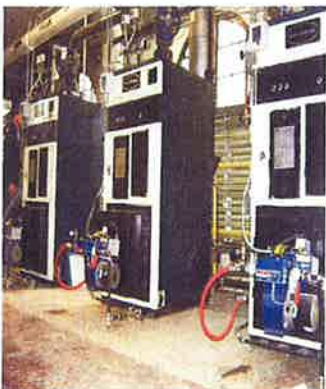
(3) WL-60 Waste Oil Boilers
