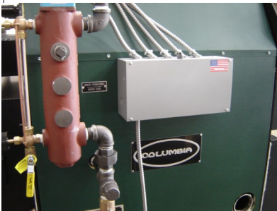
NEW MPH PANEL BOX FOR STEAM BOILERS
